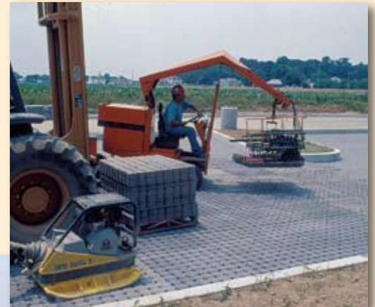
A clamp on specialized mechanical installation equipment grabs a layer of pavers for placement on the bedding. The pavers are compacted into the bedding layer, the openings and joints filled with the bedding material and compacted again to create interlock among the pavers. Since there is no curing, the pavers are immediately ready for traffic.
