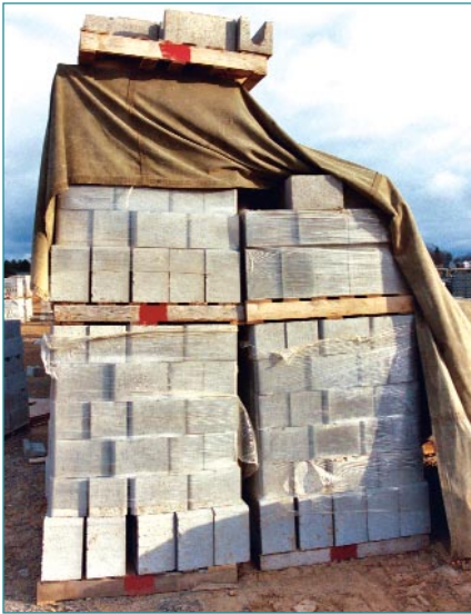
Figure 3. By placing masonry units on pallets and covering them with tarps, it is possible to keep them dry while stored at the job site. (IMG12505)
