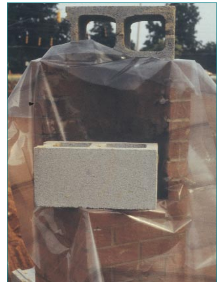
Figure 4. The top of masonry walls should be protected with a tarp whenever rain or snow is expected. It is good practice to cover work at the end of each day to help keep excessive water out and aid curing. (IMG15557)
