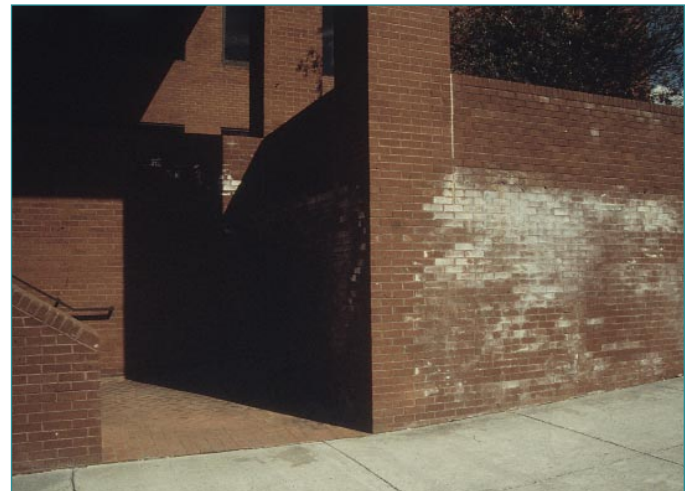
Figure 1. Efflorescence is often called “new building bloom” because it appears on fresh masonry surfaces. (IMG14593)
