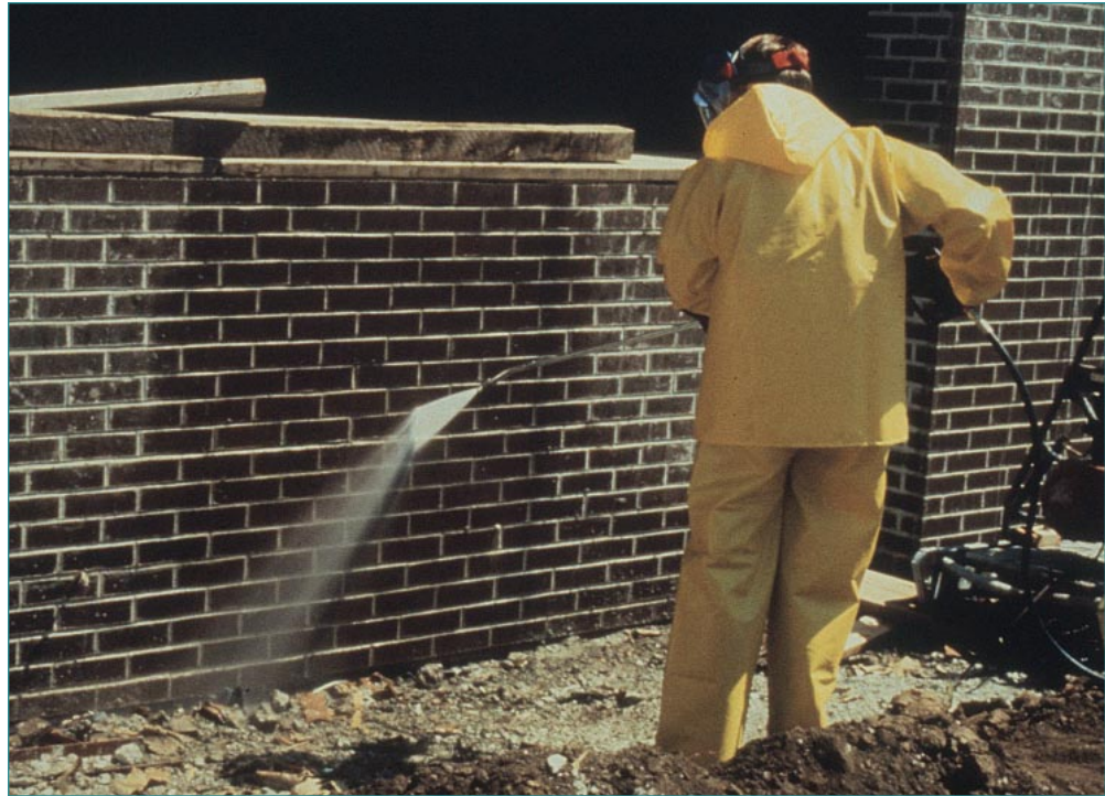
Figure 5. If efflorescence must be removed chemically, walls should be thoroughly rinsed to remove all traces of the cleaner. (IMG15558)
